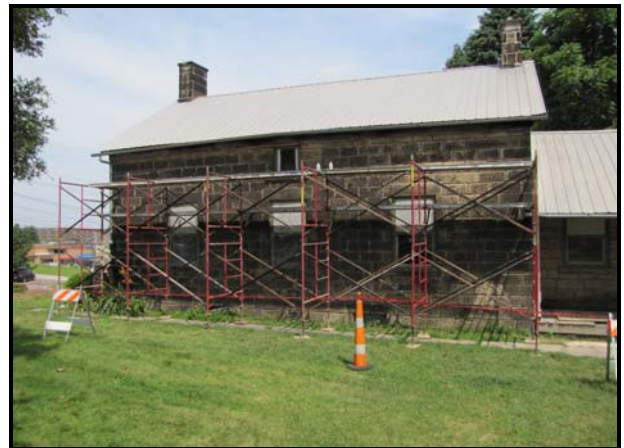
Scaffolding secured across the south side of the house for current tuckpointing initiatives
