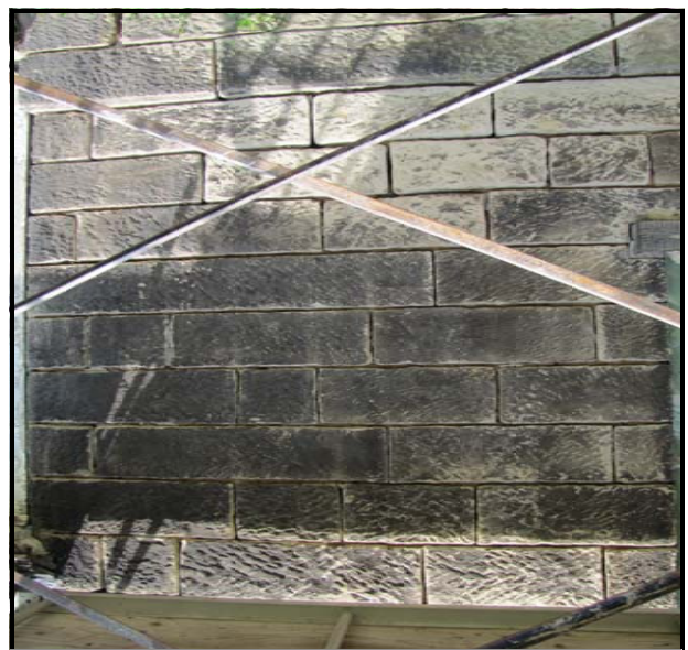
Close up of mortar joints that are first cleaned of degraded mortar, then refilled with a pre-approved custom blended mix
