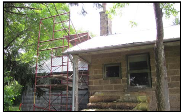
Scaffolding prepared on the north side of the house to repair adjacent chimney
